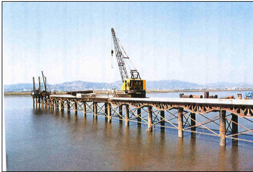
Figure 4.2 Temporary Bridge will be constructed for the movement of vehicles and machinery
