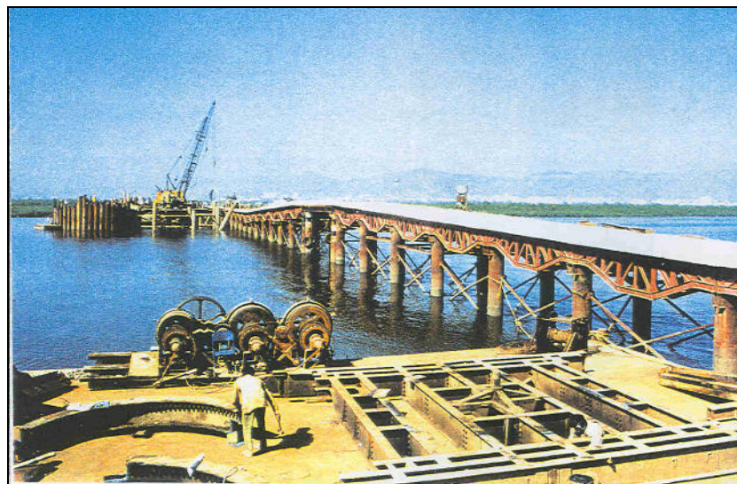
Figure 2.5 Temporary Bridge to be constructed in the Mudflats to avoid disturbance of Mudflats
