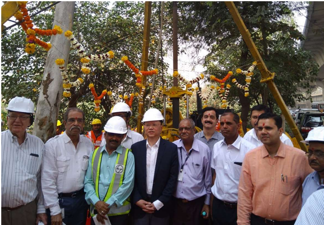
Package-1 GTI Works Start at Sewri Interchange at BP-7 in Ramp B
