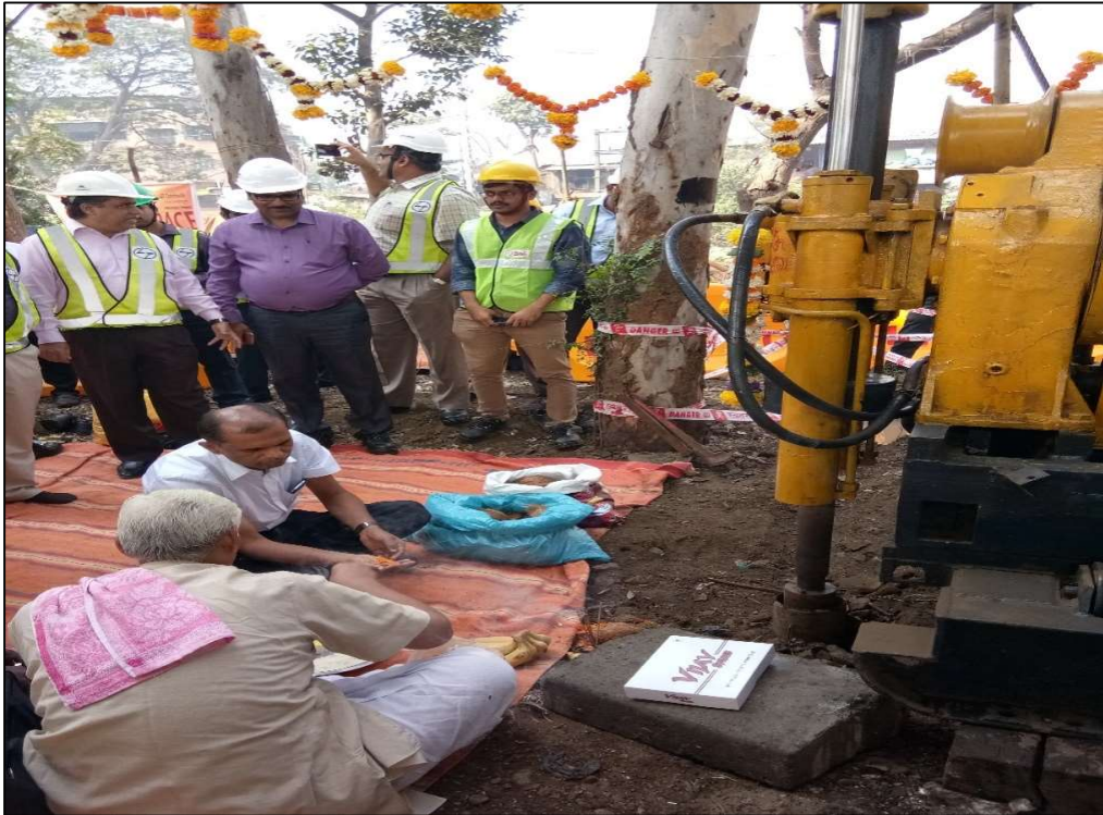
Package-1 GTI Works Start at Sewri Interchange at BP-7 in Ramp B
