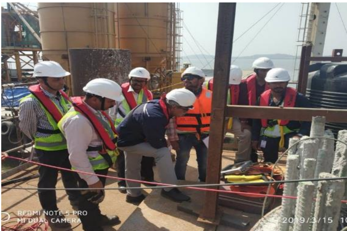
Photo No. 18: Cross Hole Sonic Logging Test at MP 162/02 RHS location in progress
