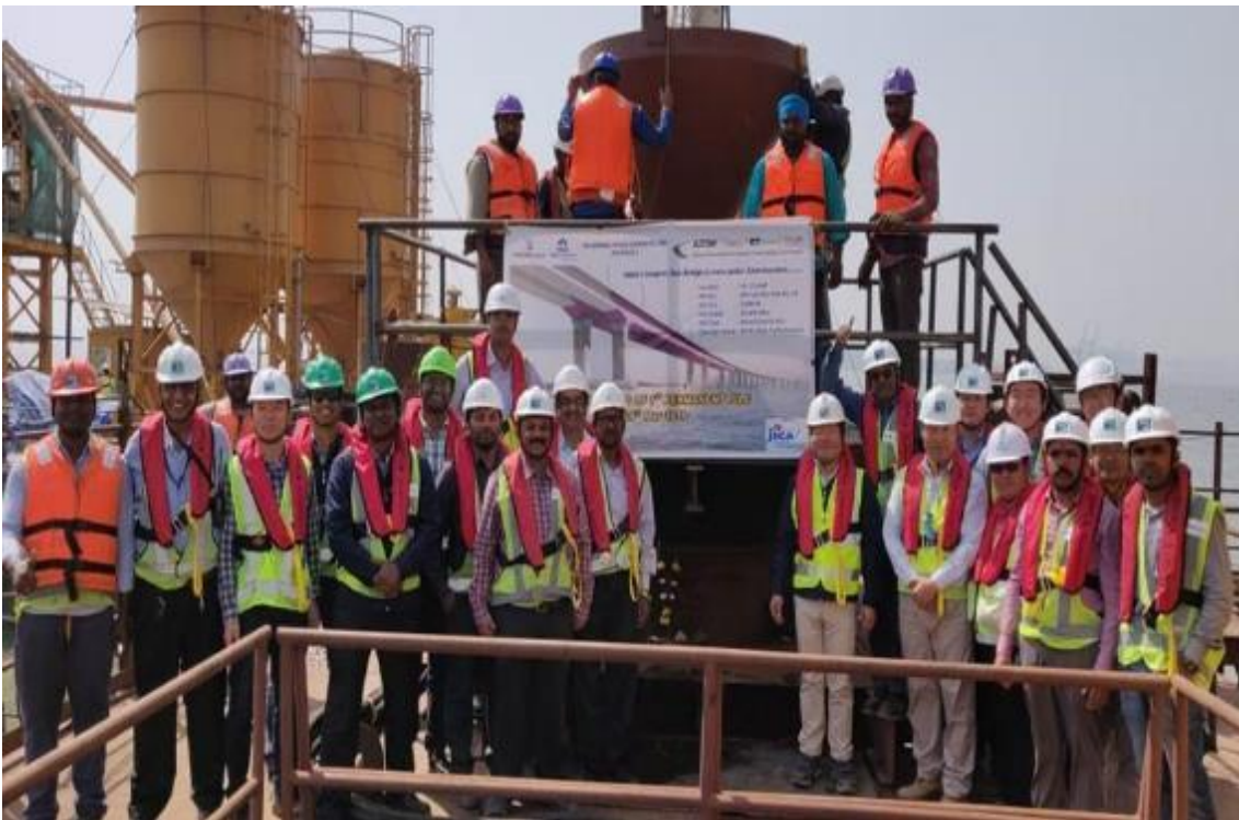
Photo No. 24: A group Photo Taken after first Permanent Pile Concreting done at the Marine Location
