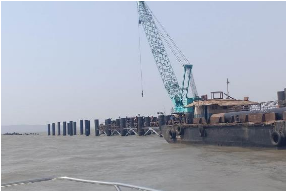
Photo No. 19: Fixing of bracing works at Temporary Bridge Front-2 at MP 214 in progress
