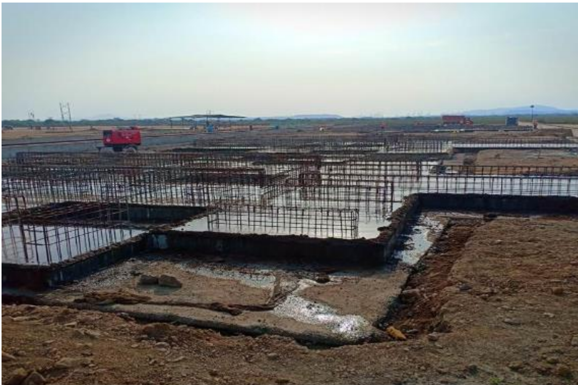
Photo No. 22: Mould Foundation Curing Works at Casting Yard Bay-2 in progress
