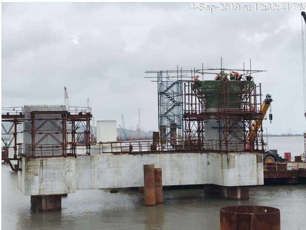
Photo No. 4: Pier cap reinforcement work at MP 06 N is in progress
