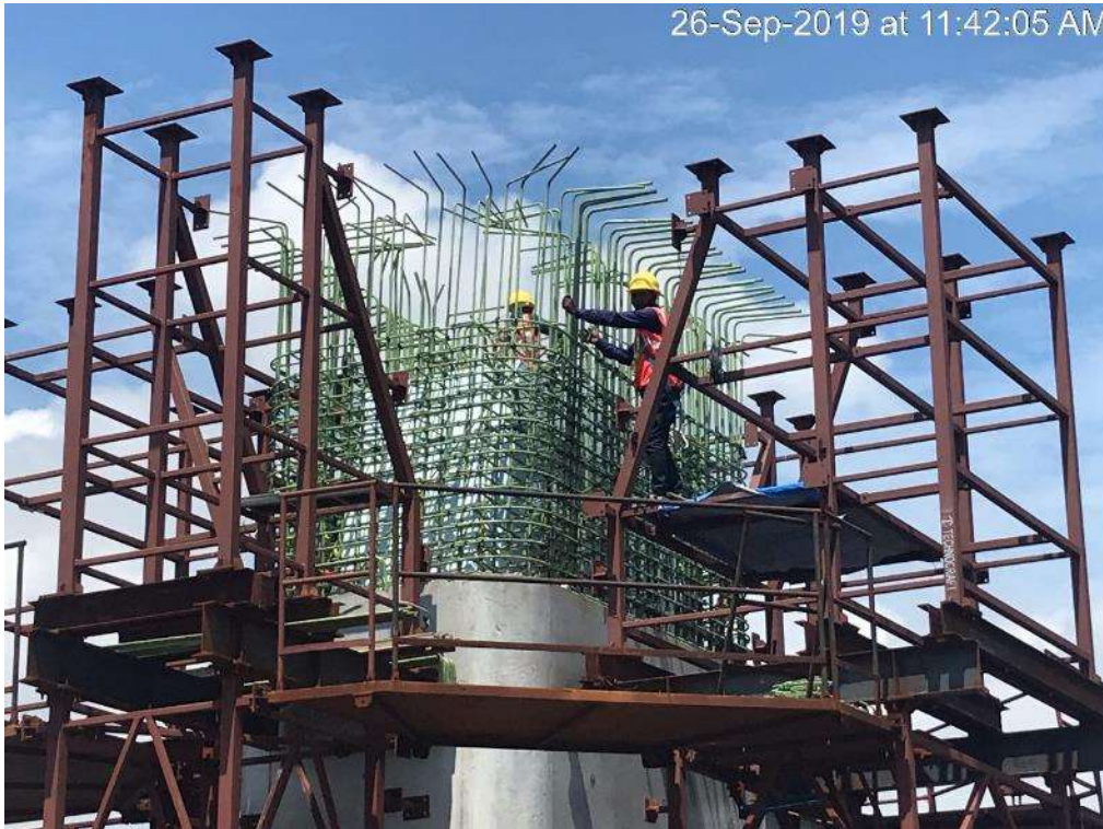
Photo No. 3: Pier Cap reinforcement work at MP 06 N is in progress
