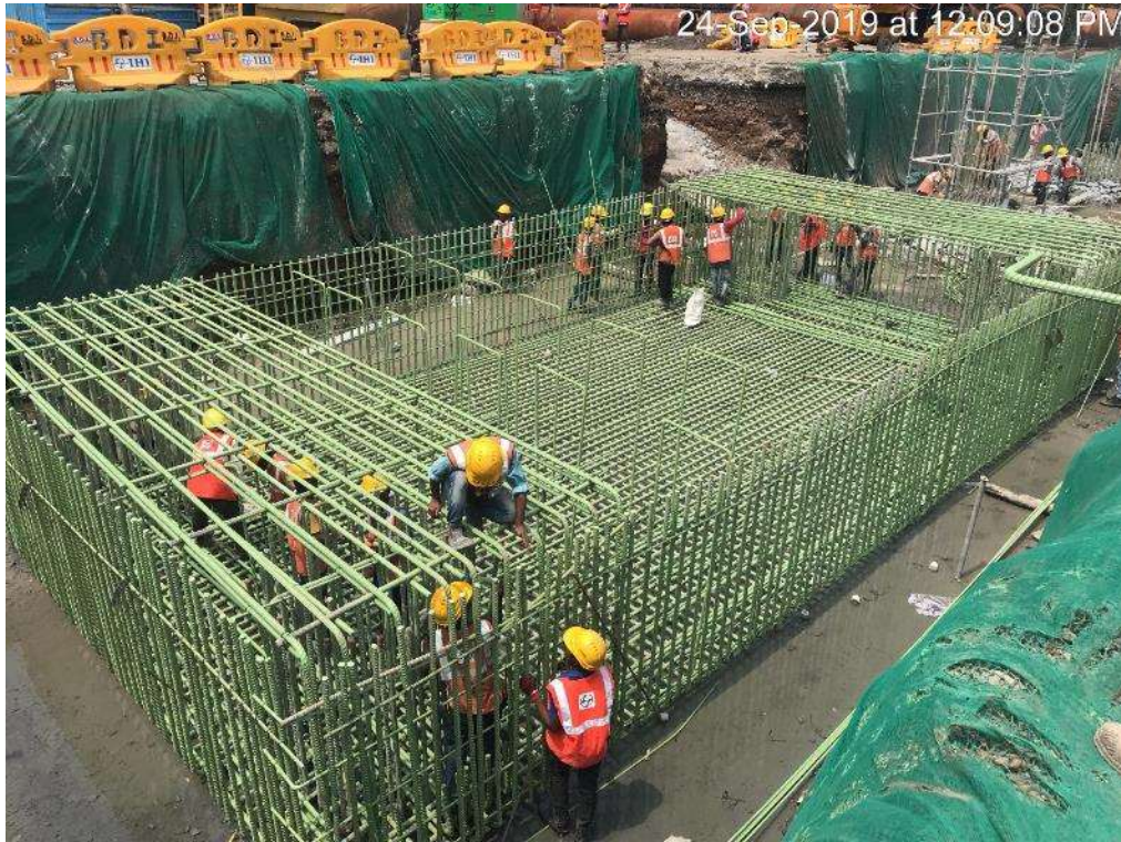
Photo No. 5: Pile Cap reinforcement work at BP 50 Interchange location is in progress
