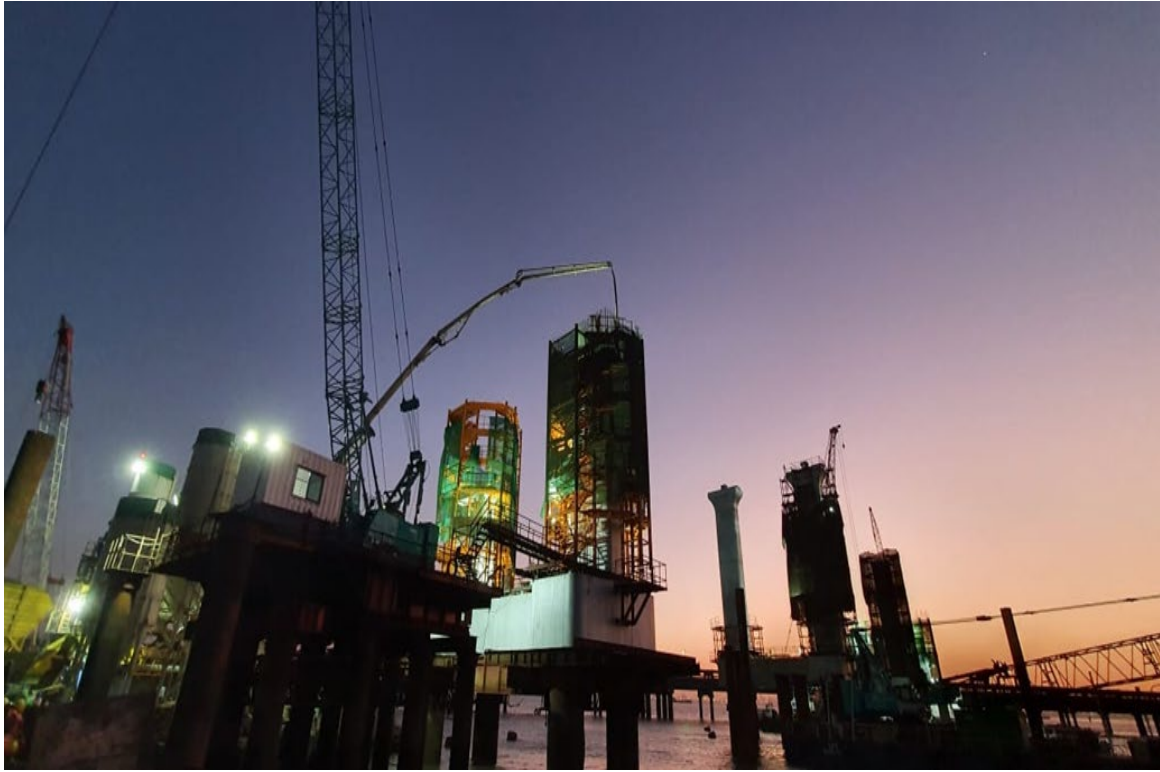
Photo No. 1: MP 84 N Pier Concrete – Marine Area
