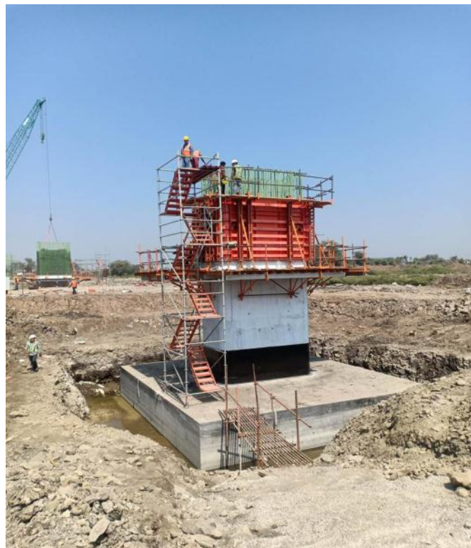
Photo No. 12: Pier final lift formwork inspection at MP 243 LHS in progress
