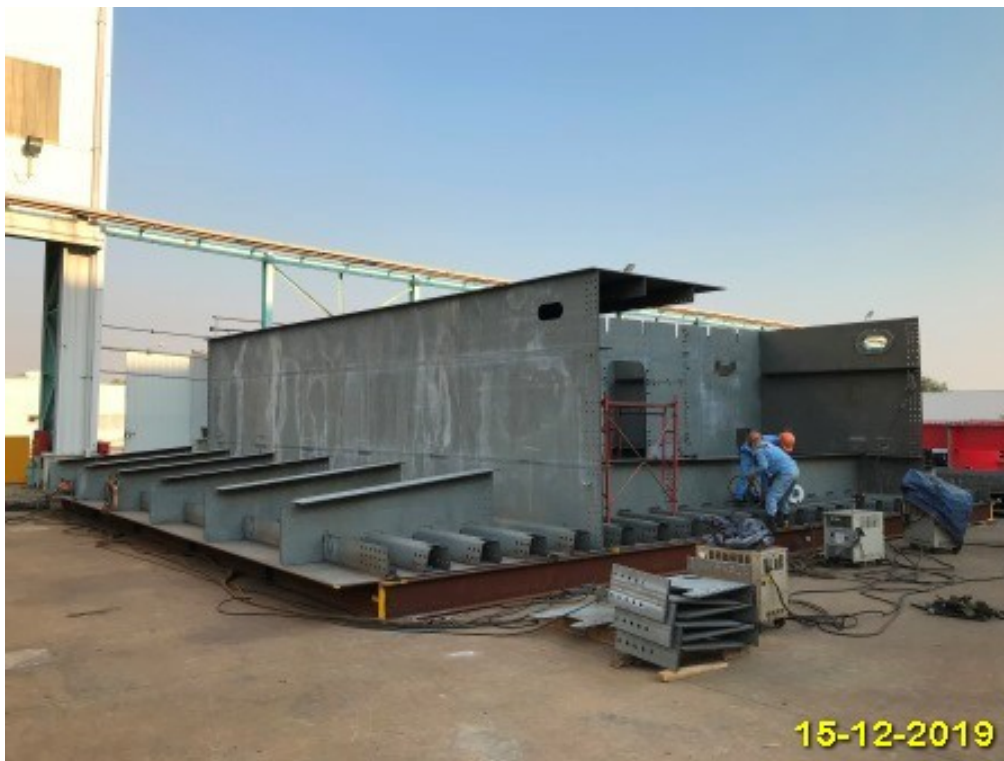
Photo No. 12: Segment assembly for OSD Girder Fabrication OS01-NG (lot1) -IIA, Vietnam
