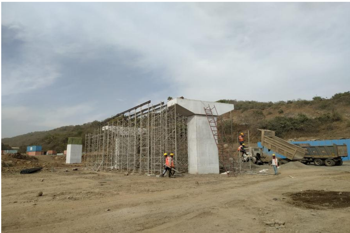
Photo No. 12: Span MJP-07 to 08 (Chirle Ramp) Staging for cast in-situ voided slab in progress
