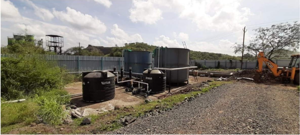
Sewage treatment plant at labour camp
