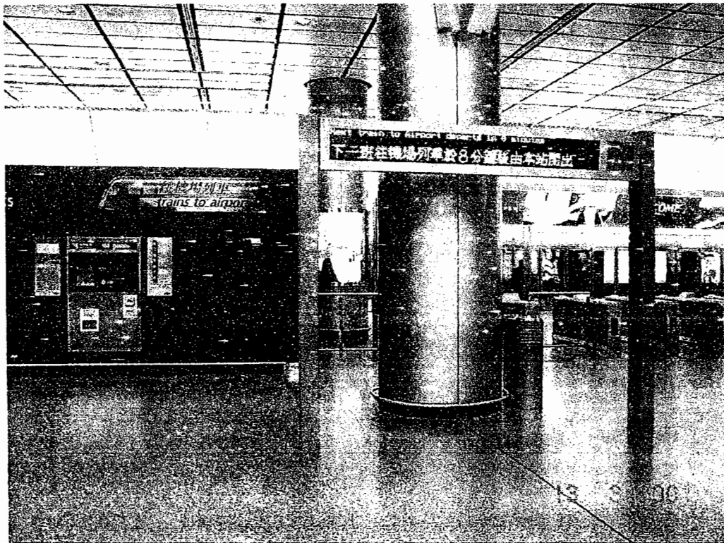
PIDS at Concourse
