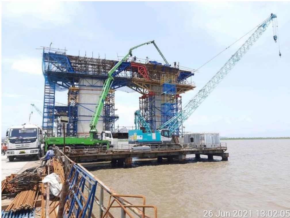
Photo No. 6: Integral Pier head segment concreting at MP 222 RHS in progress
