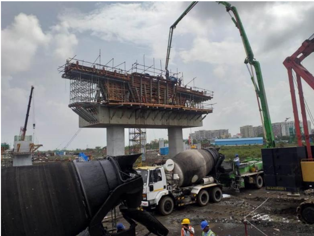
Photo No. 10: Large Pier head segment concreting at MP 256 RHS in progress
