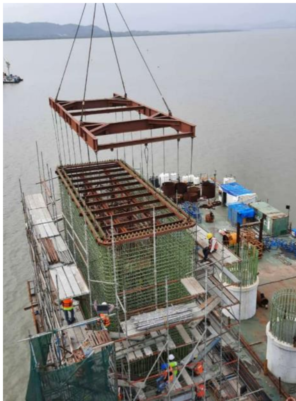
Photo No. 10: MP 125 3rd Lift Pier Prefab Reinforcement at Marine Section in progress
