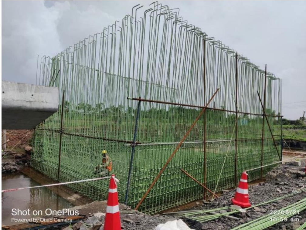
Photo No. 7: Retaining wall raft reinforcement tying at Ramp MA in progress
