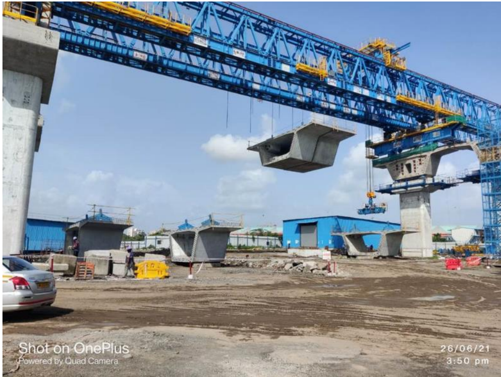
Photo No. 5: LG-3 Winch Load test at Span MP 265-264 LHS in progress
