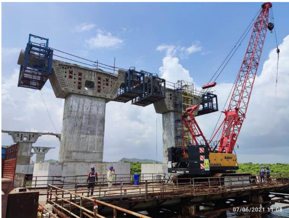
Photo No. 12: PT strands threading works at MP 232 LHS and RHS in progress
