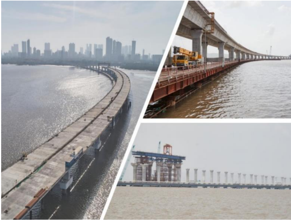
Photo No. 1: A view of MTHL Bridge taken from the Interchange Section looking towards the sea
