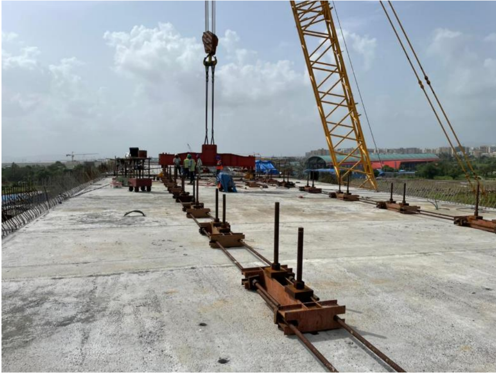
Photo No. 11: Span RMP 280 to 281 - segment gluing and temporary stressing work in progress
