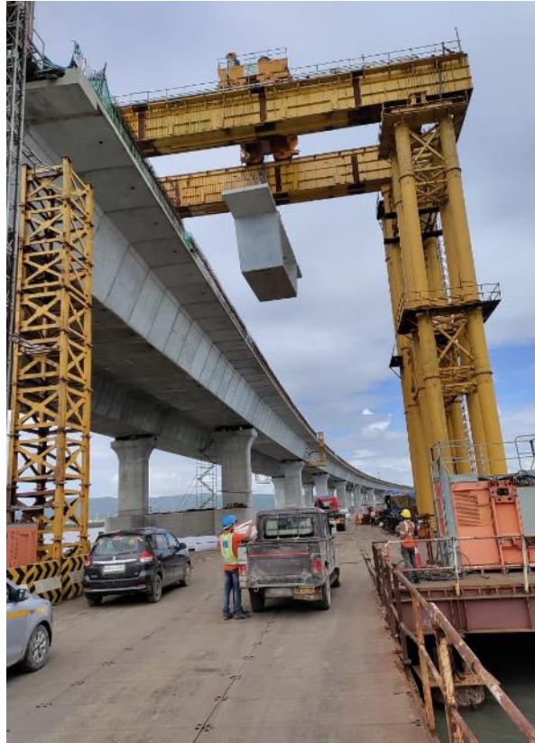
Photo No.7: Segment Lifting By Feeding Portal Arrangement - Intertidal Section in progress
