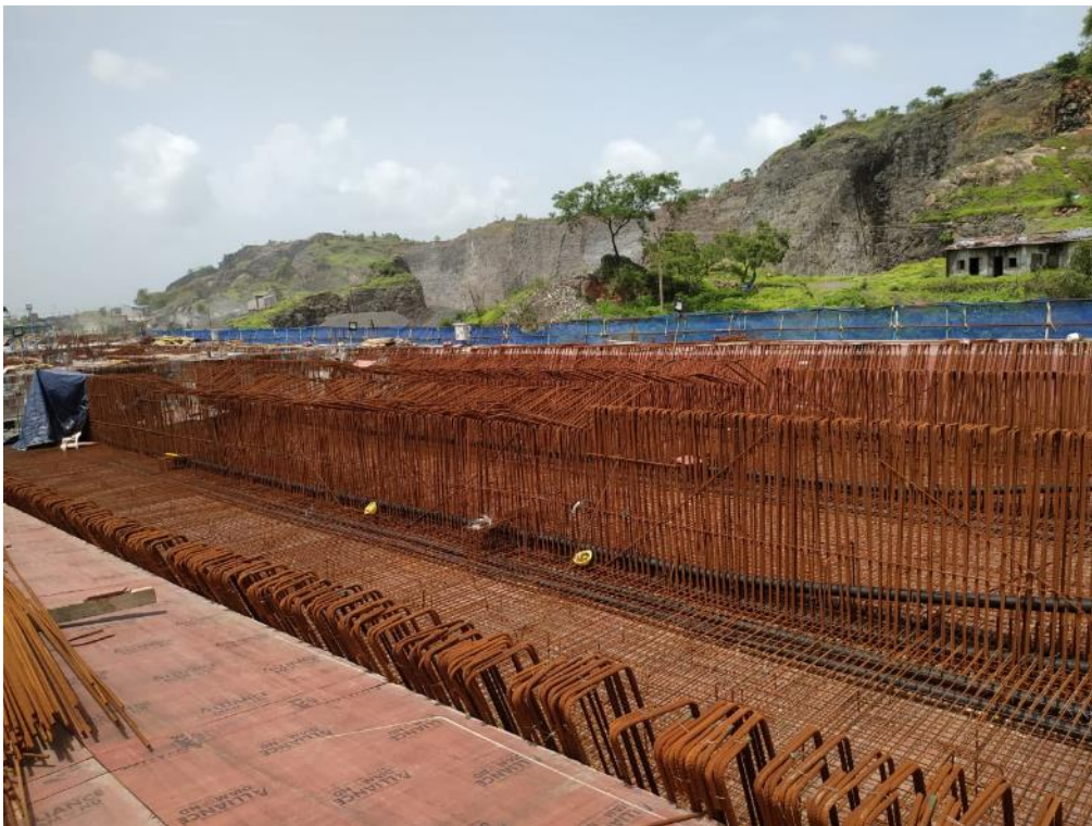
Photo No. 8: Cast in situ three cell box girder Span RP02-01(Jasai) bottom soffit slab reinforcement & profile in progress
