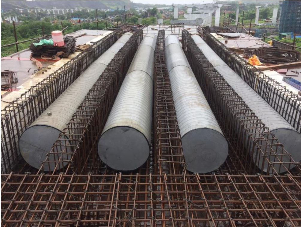
Photo No. 7: Voided slab Span JMP16-17 during bottom soffit reinforcements inspection in progress
