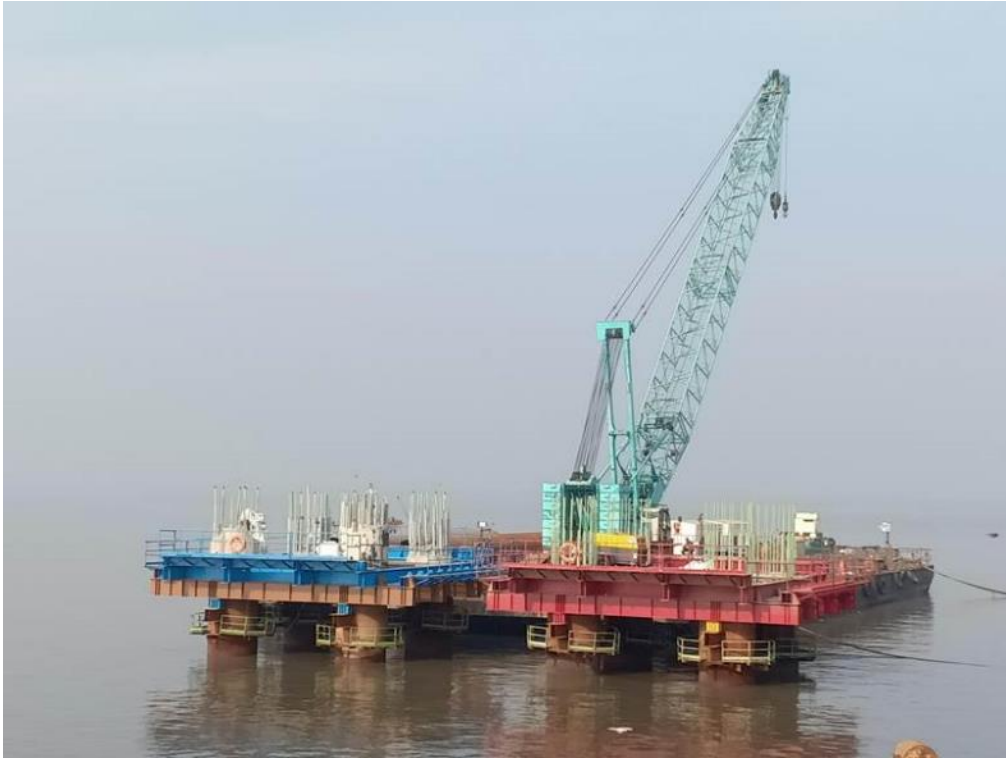
Photo No. 3: Pile Cap bottom formwork and Pile head chipping in progress at MP 206 LHS and RHS in progress
