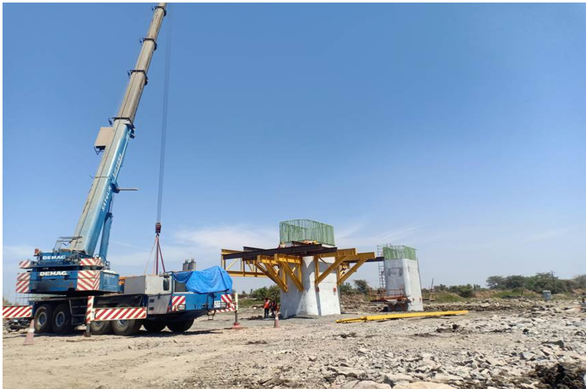
Photo No. 10: Bracket fixing for Pier Cap at MP 243 RHS in progress
