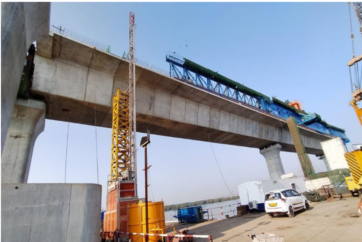
Photo No. 10: Segment Erection by LG at MP 14-15 N11- Intertidal Area is in progress
