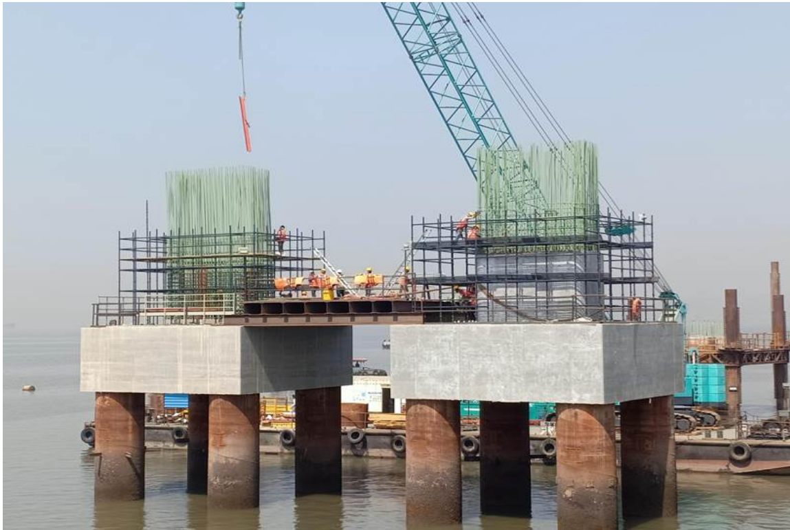
Photo No. 5: Pier 1st and 2nd lift reinforcement tying in progress at MP 206 LHS and RHS
