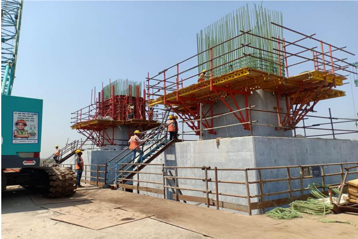
Photo No. 7: Pier 2nd lift formwork and 2nd lift reinforcement at MP 231 RHS and LHS in progress
