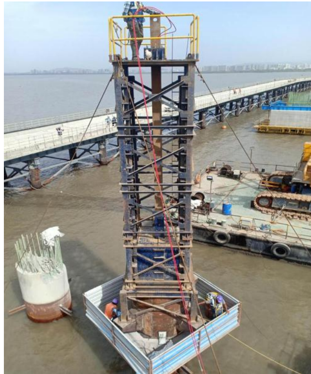
Photo No. 4: High Strain Dynamic Pile Load Test at MP 209/02 LHS in progress
