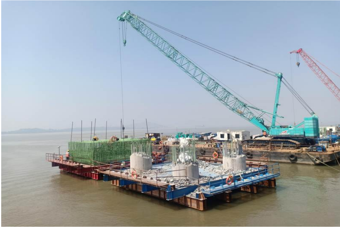
Photo No. 3: Pile Cap Reinforcement and Pile Head Chipping at MP 207 LHS & RHS in progress
