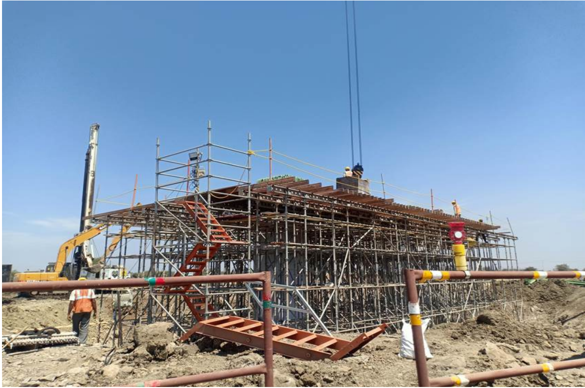
Photo No. 9: Scaffolding and Bottom formwork for Portal Beam at MP 245 LHS in progress
