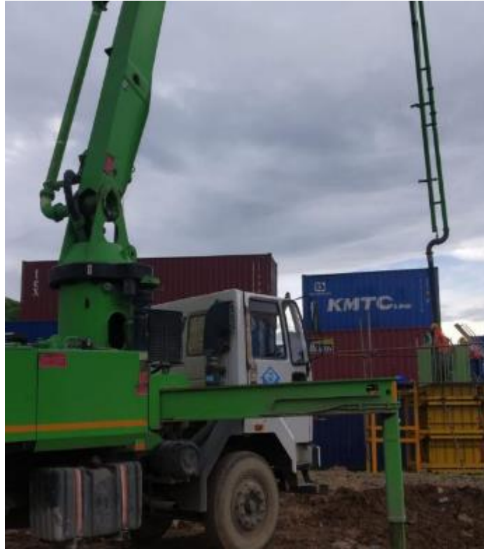
Photo No. 7: Final lift concrete pouring at Pier No. PMP-13 (Chirle) in progress
