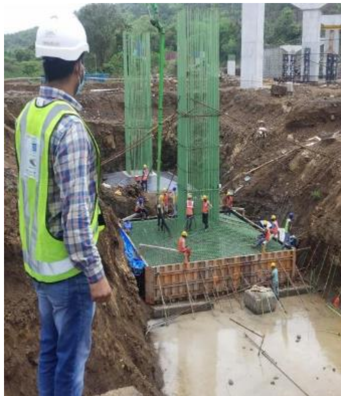
Photo No. 4: Concreting Works at Foundation No. LP 38 at Chirle in progress
