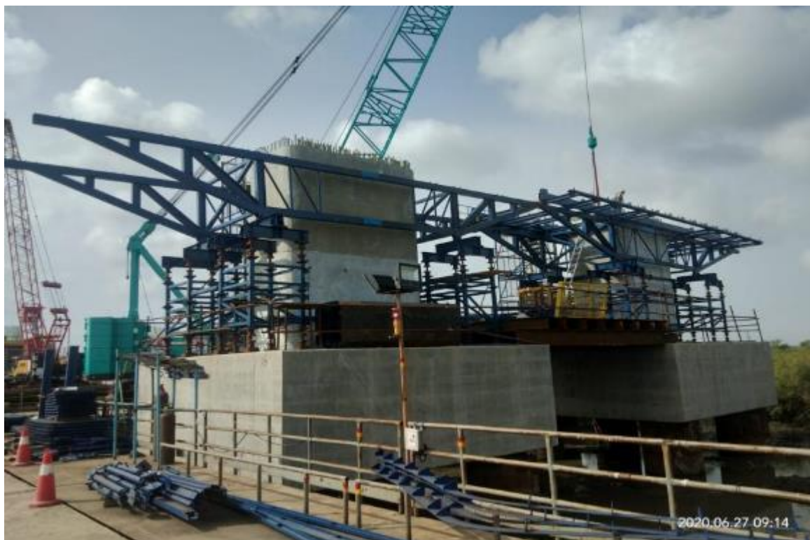
Photo No. 4: Formwork for Pier Head Segment at MP 237 LHS and RHS in progress
