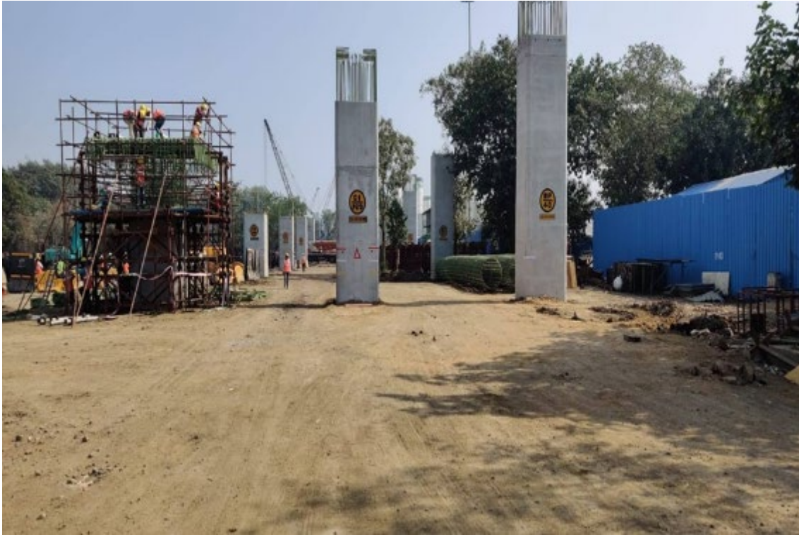
Photo No. 1: C2P9 S Pier Head Reinforcement Works at Interchange in Progress
