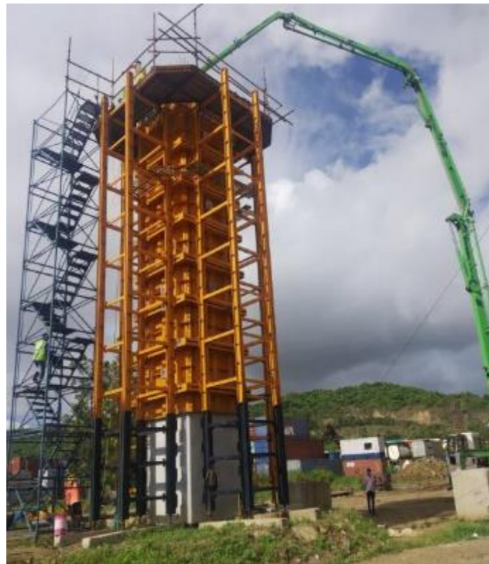
Photo No. 8: Final lift (8.135M) concrete pouring AT Pier No. LP-31 (Chirle) in progress
