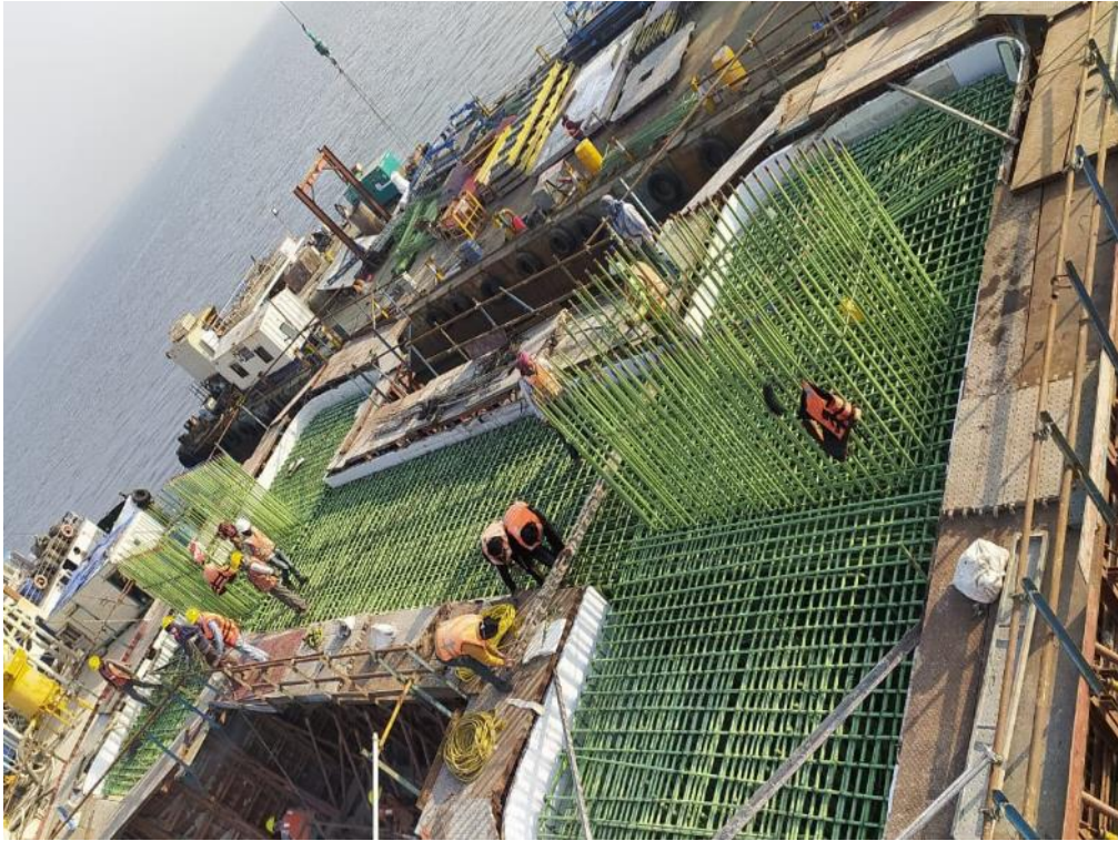
Photo No. 9: MP 123 Pile Cap Pre-Pour Checking at Marine Section in progress
