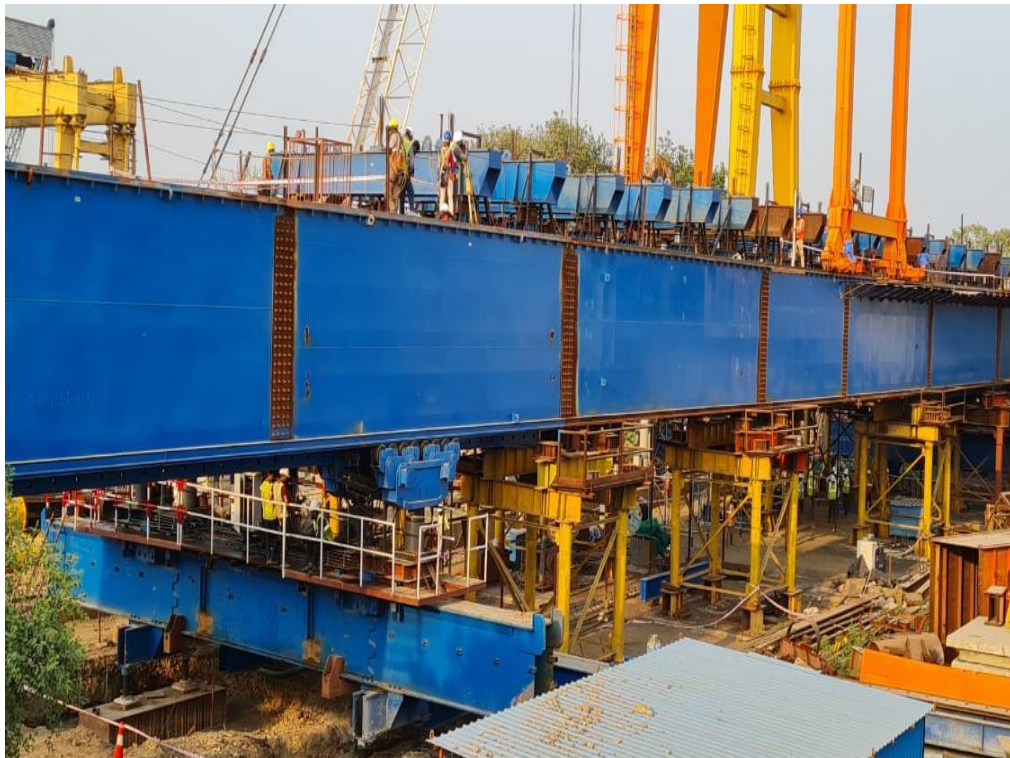
Photo No. 4: LG-3 Load Test at the Precast Yard Location in progress
