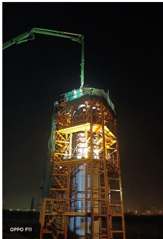
Photo No. 2: MP44S L2 (Final Lift) Pier Concrete Works – Intertidal Location in progress
