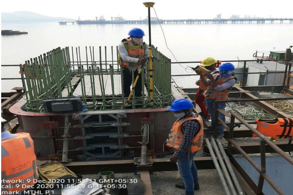
Photo No. 11: MP 97 S Starter Co-Ordinates Checking at Marine Location in progress
