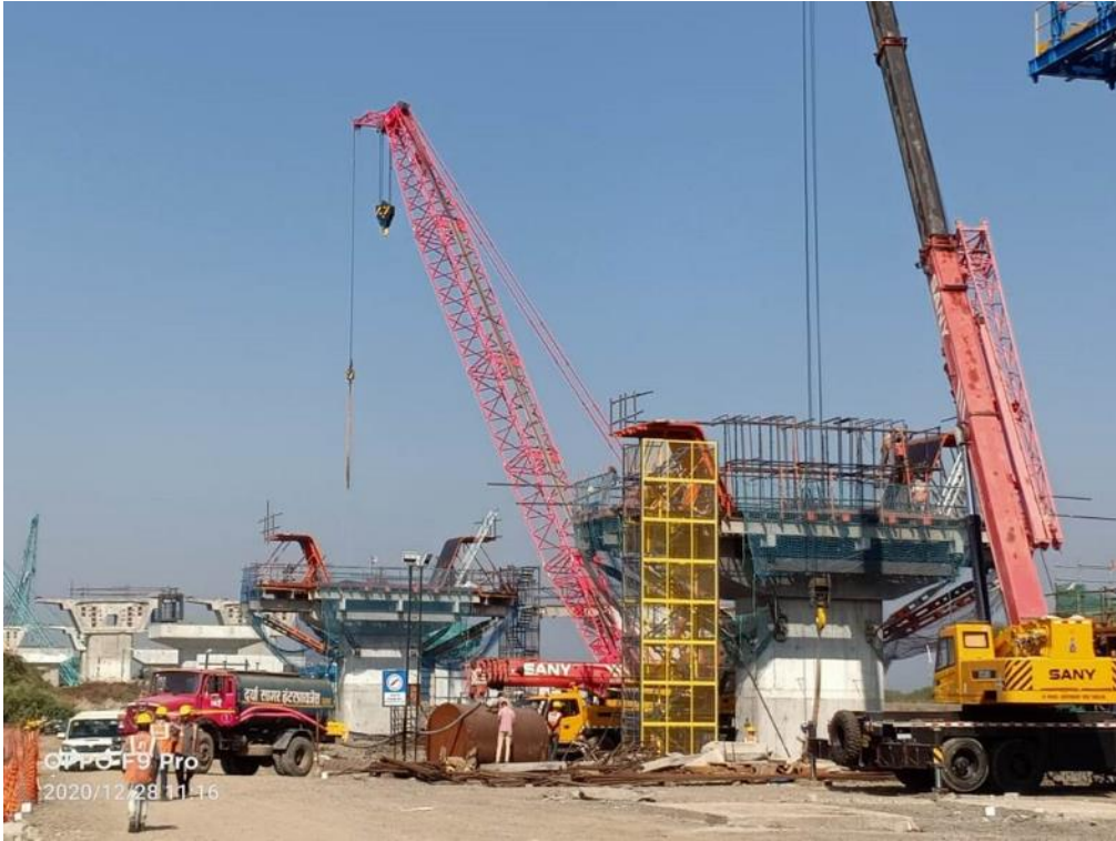
Photo No. 5: Pier head segment reinforcement tying at MP 242 LHS in progress
