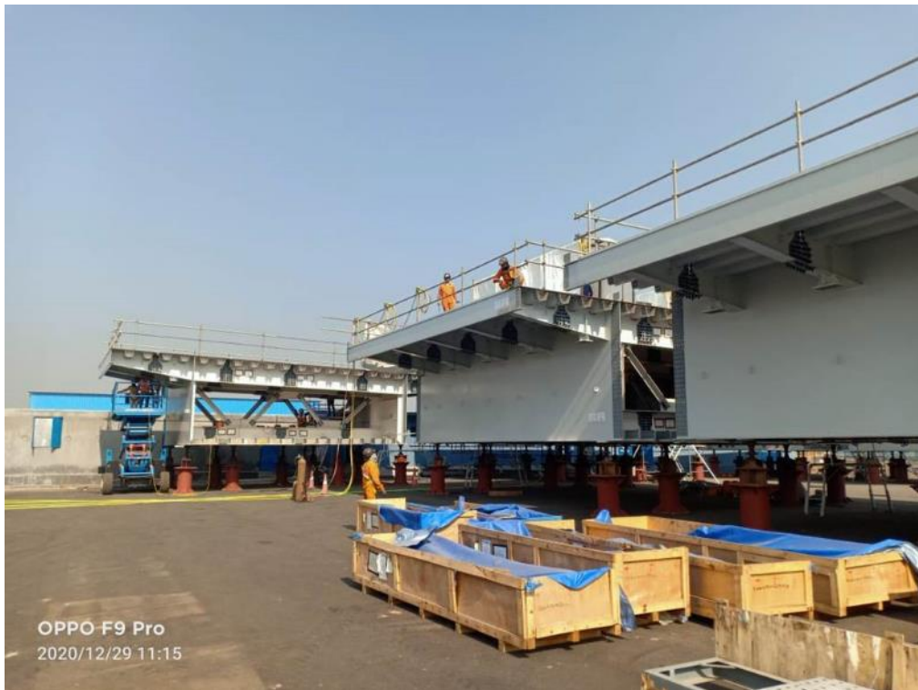
Photo No. 4: OSD small block assembling and welding at Karanja Port in progress
