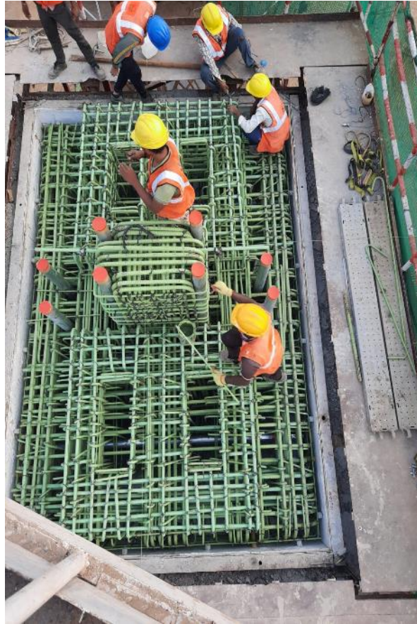
Photo No. 3: LP 6 N Pier Head Pre-Pour Checking - Interchange Location in progress
