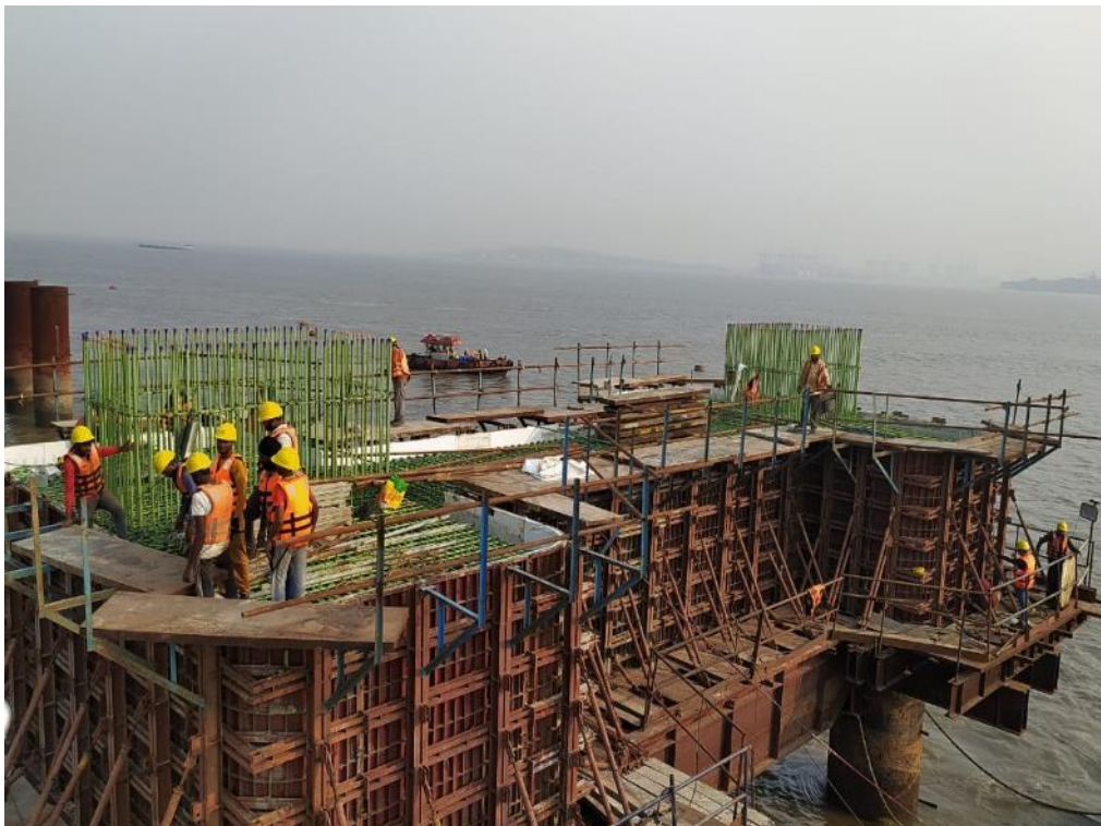
Photo No.8: MP 120 Pile Cap Pre-pour Checking at Marine Section in progress
