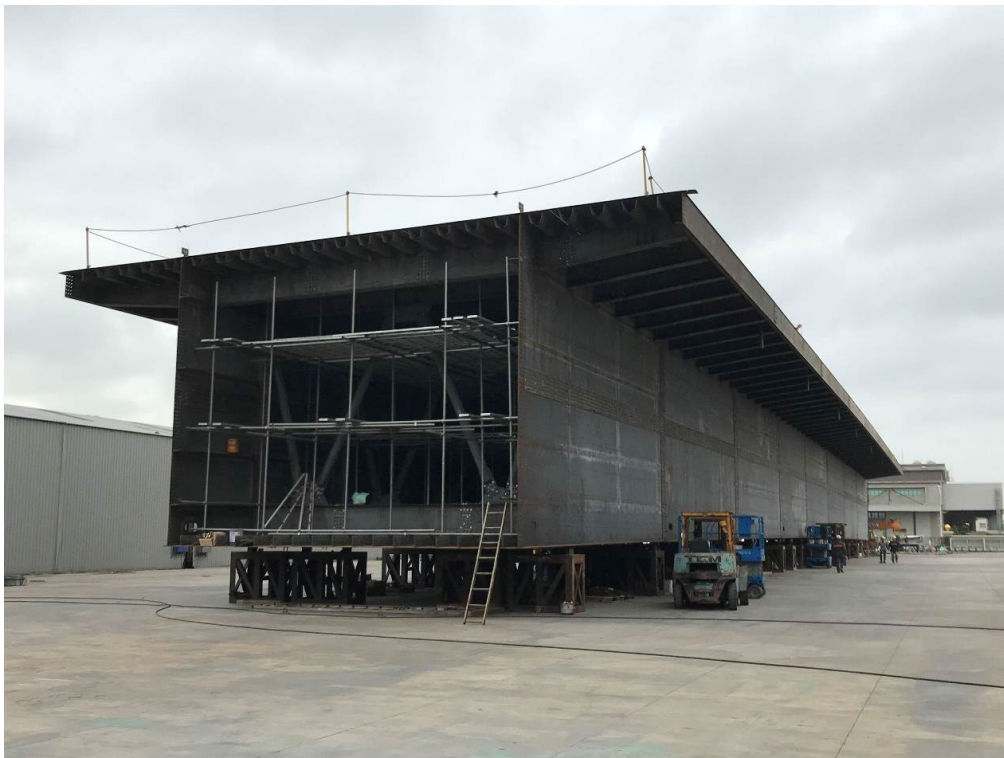
Photo No. 12: Trial Assembly completion for OSD Girder Bridge P1-OS01-SG (Lot5) / Seg. 12~17 Steel Bridge Fabrication Progress: At Ta Chang Tsoo Industrial Co., Ltd. (TCT)-Taiwan
