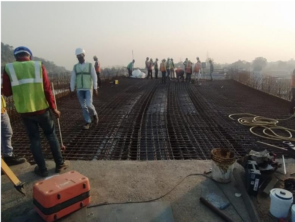
Photo No. 8: voided slab and cantilever portion reinforcement at Span MJP6 - MJP7 in progress
