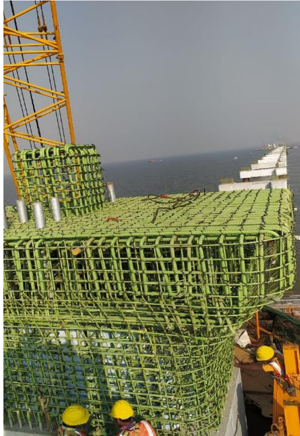
Photo No. 5: MP100 S Pier Head Rebar Inspections at Marine Section in progress
