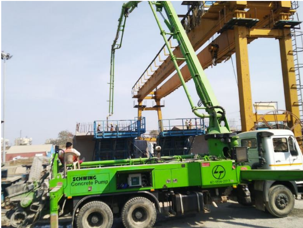
Photo No. 9: PCY Bay 1, Segment K-55 Span LMP 280-281 Concrete pouring in progress
