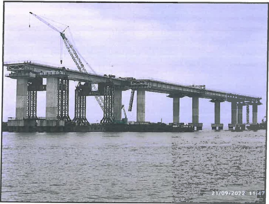
Photo No. 10: 7th OSD span erection at Span MP 178-179 LHS in progress
