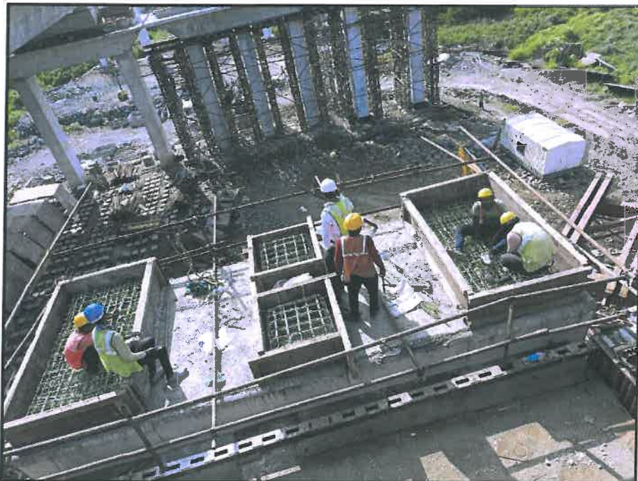
Photo No. 8: Chirle Pier cap LP 30 pedestal & seismic arrester pre-pour inspection works in progress
