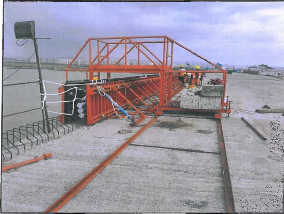
Photo No. 3: Outer Crash barrier formwork alignment at Span MP 222-223 LHS in progress
