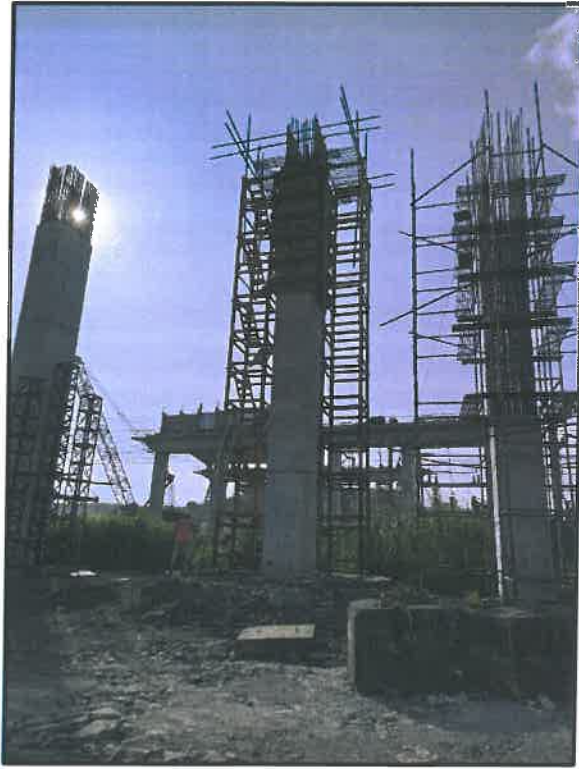
Photo No. 7: Chirle Pier RP 28 L final lift shuttering works in progress
