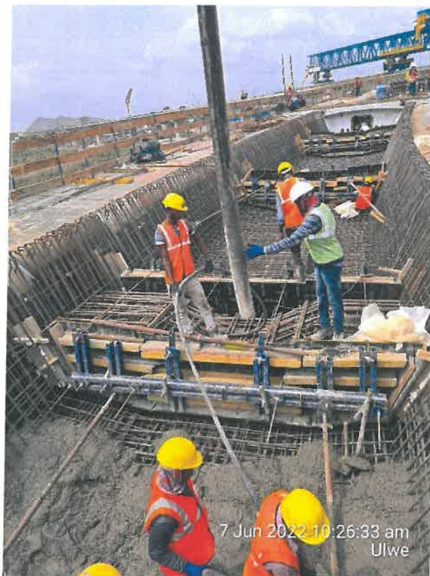
Photo No. 7: Cast in situ slab concreting at Interchange Area in progress
