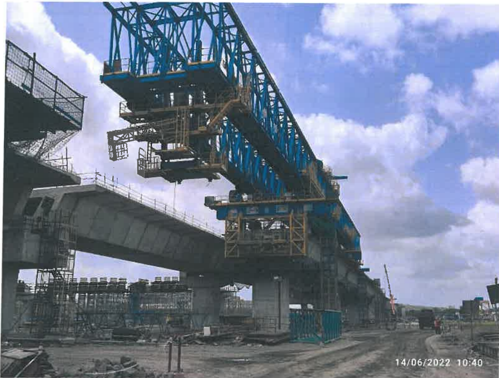
Photo No. 1: LG-3 Wet joint formwork fixing at Span MP 253-255 RHS in progress
