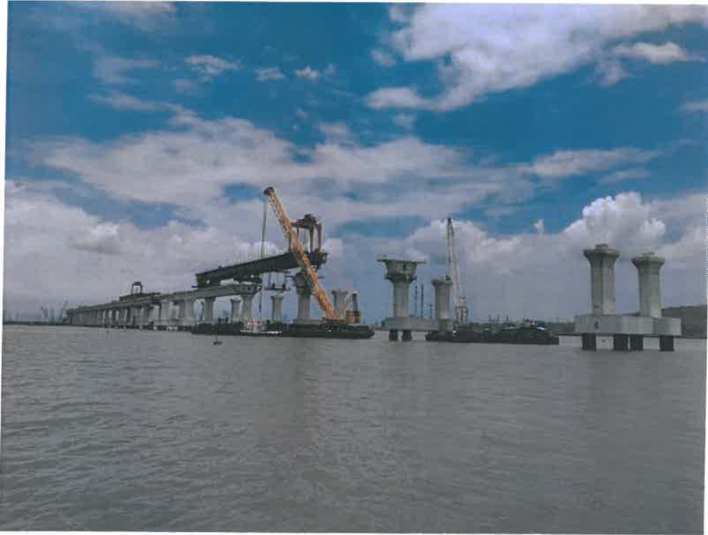
Photo No. 1: LG- 3 Span Erection at Marine Location looking towards Navi Mumbai
