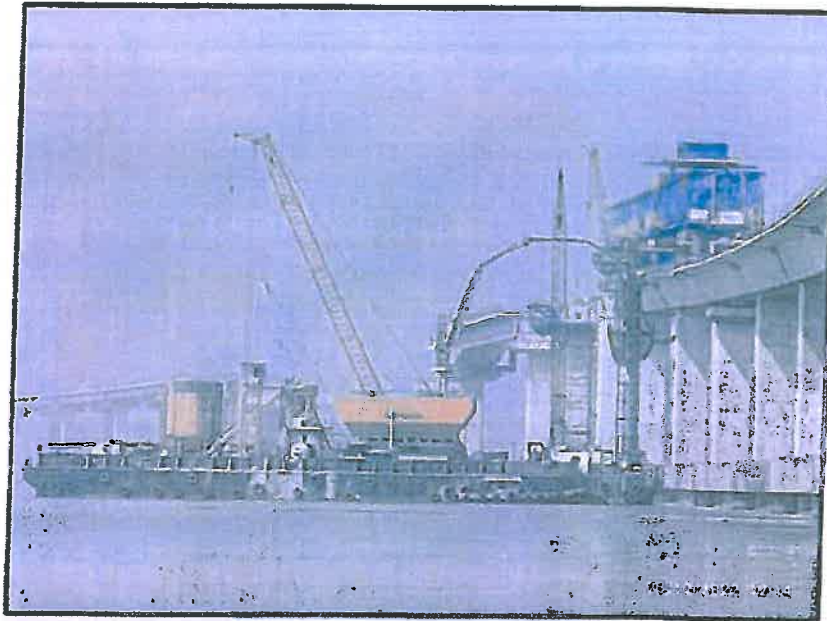
Photo no.3- Pier final lift concreting in progress at MP 191 RHS Substation.
