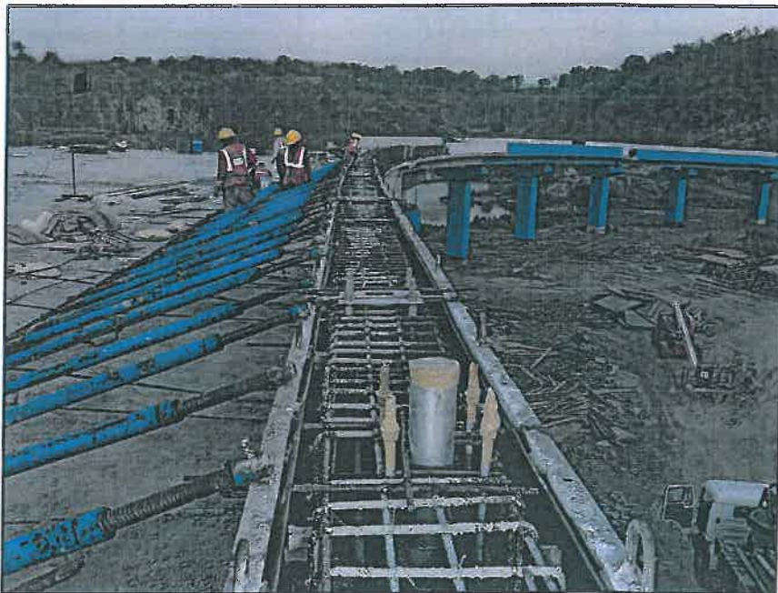
Photo no.4- A Outer crash barrier shuttering work at Chirle span RP36-37.t-grade location.
