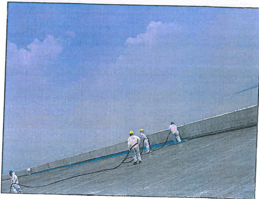
Photo no.2- Preparatory works for 26 th OSD erection in progress at Span MP 173-173A LHS.
