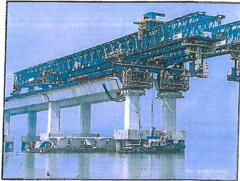
Photo no.12- Wet joint formwork in progress at span MP 152-153 RHS and segment lifting in progress at span MP 152-153 LHS.
